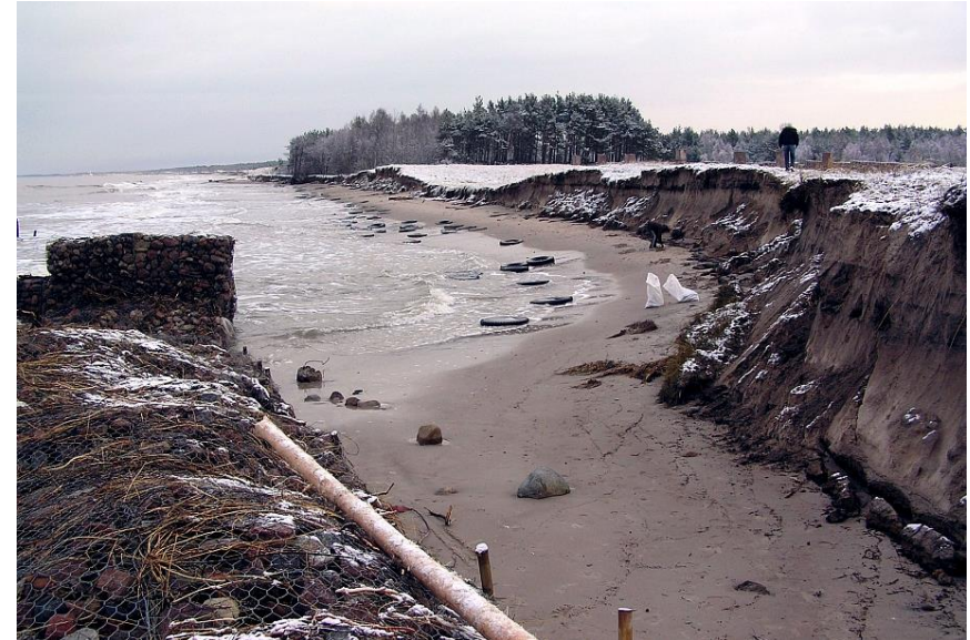
Coastal erosion outlined after storm surge (2018, LSM)
